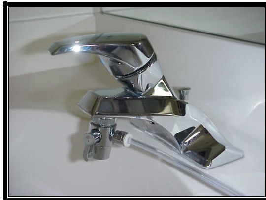
Portable Water Feed Sink Hook-Up
